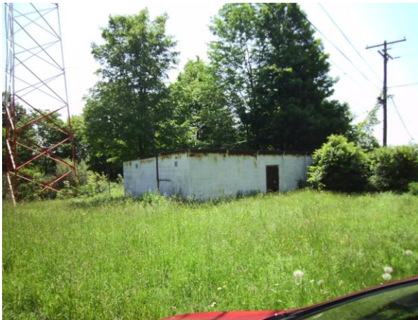
Poorly Maintained Site
